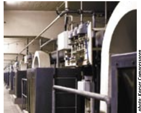
photo: Kaeser Compressoren
