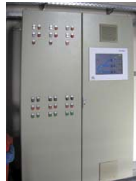
The control cabinet in the valve chamber – only the Kontron flat-screen points to the hidden PC intelligence of the ThinkIO behind the doors.
