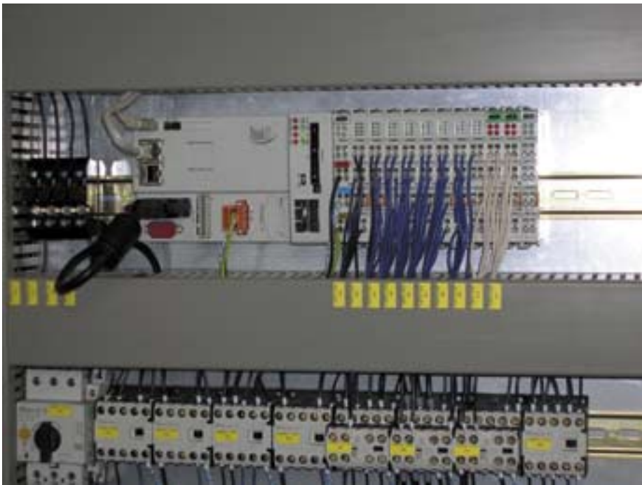
Controlling cabinet, including the complete PC.
