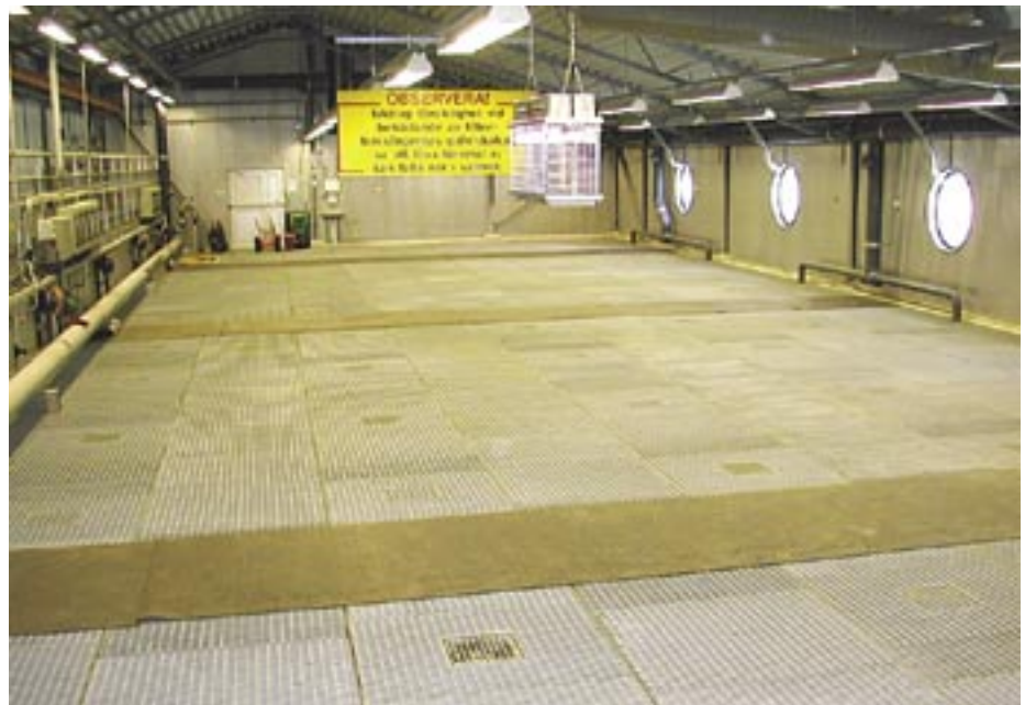
The filter hall at Växjö treatment plant.
