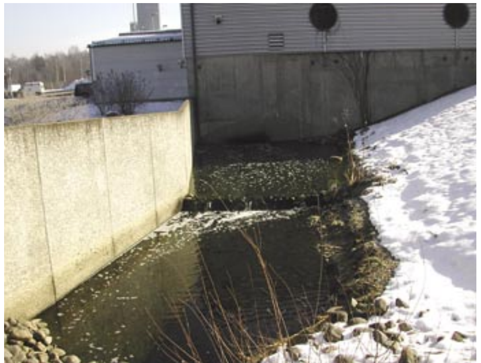
The outlet from the Växjö treatment plant.
