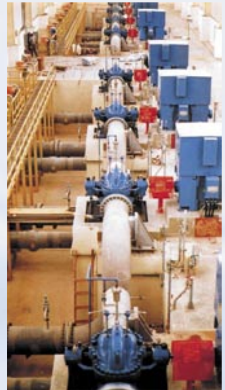
Fig. 2: Experienced pumping station designers can obtain the highest possible level of efficiency by selecting a suitable number of pumps and an appropriate rotation speed.
