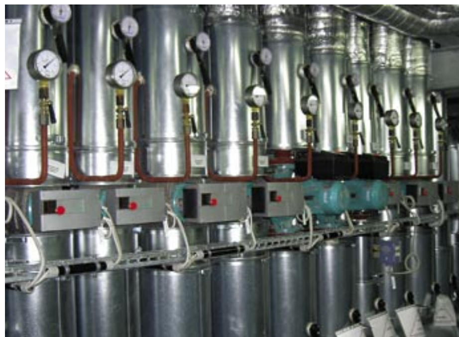
The high-efficiency pumps applied in heat supply consume more than 80 % less power compared to uncontrolled pumps. The redundantly installed main pumps of the “Wilo-VeroLine IP-E” type are automatically adjusted to different load states with a built-in frequency converter which allows for energy savings of up to 50 %.
